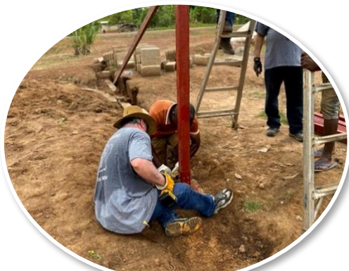
Helping a local Pastor secure the framework. There is power in teamwork!
